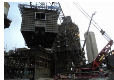
Fig.23 Fabric Filter is lifted up on its way to take the Gravel Bed Filter place
