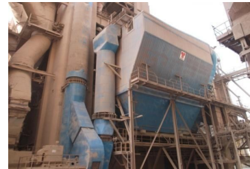
Fig.15 The converted bypass filter after conversion into FF in Tourah cement Co. (December 2011).
