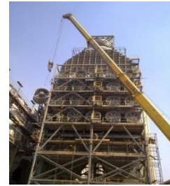
Fig.21 Heat Exchanger before FF at Cooler area
